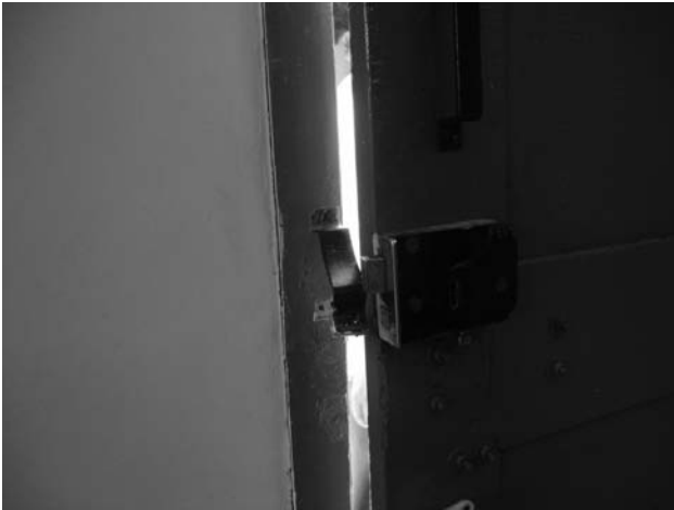
Fig. 2. The door was broke open from outside.
